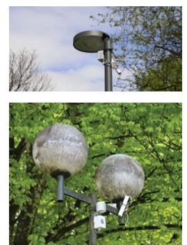
Climate sensors installed on street lamps
